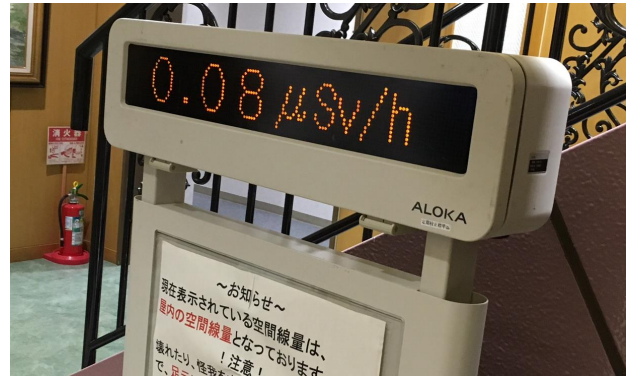
Figure 3. Radiation counter in the hotel, Naraha town
